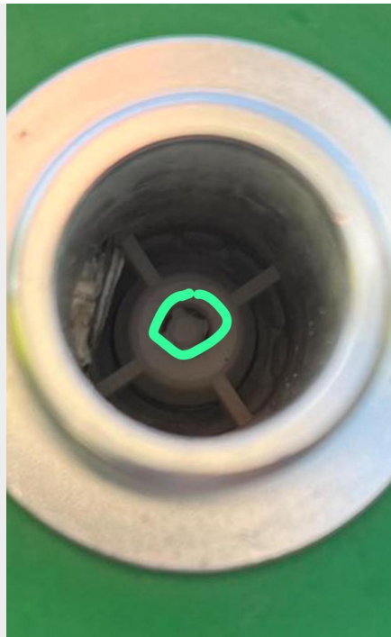
Valve on outlet port on chiller
